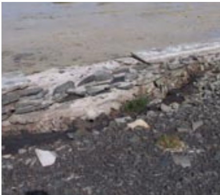
Repairs required to sea wall
