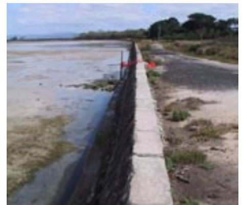
Poorly defined track on foreshore edge
