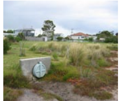
Flood gate on drainage system to control tidal inflow
