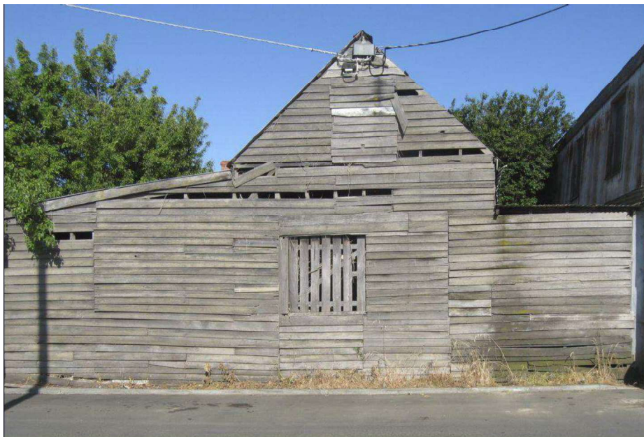
Figure D7. A timber outbuilding remains on the east boundary, which is an early stable (date not confirmed). It has a gabled roof with a filled in opening in the gable end, and another one below, and skillion additions off the long elevations.
