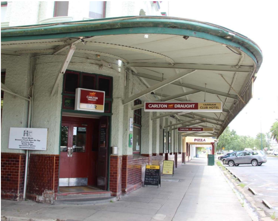
Figure D3. The wide cantilevered verandah runs across the facade and returns on part of the north elevation, with large rounded corners. It has corrugated iron cladding (overpainted) to the roof and retains the original metal support structure underneath. The ground floor has glazed brown tiles to the dado level with roughcast render to the top 2/3 of the wall (overpainted).
