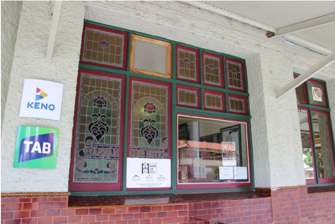
Figure D5. This photo shows the leadlight window group to the south (right) of the northern corner entrance. This is the only altered opening to the facade, as it originally had an entrance door in the right half (since closed over sympathetically). The leadlight to this window contains the words 'YARRAM CLUB HOTEL'.
