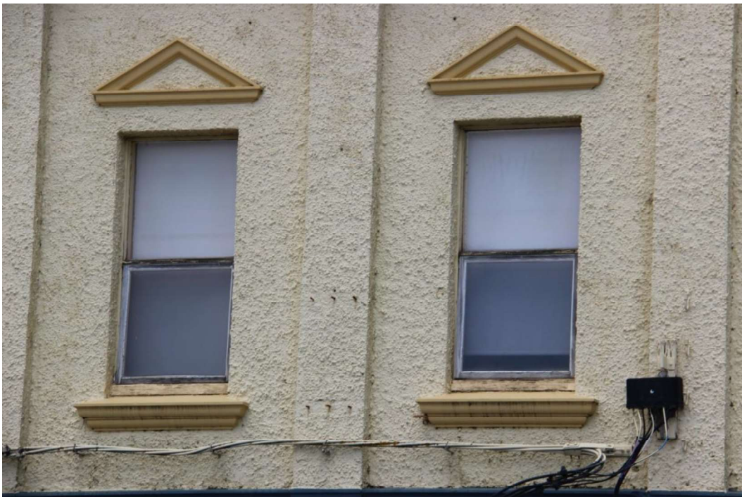
Figure D2. A single window appears in each bay (formed by the pilasters) to the first floor. The windows are one-over-one timber sashes with a moulded sill and moulding above that forms an abstracted Classical pediment.
