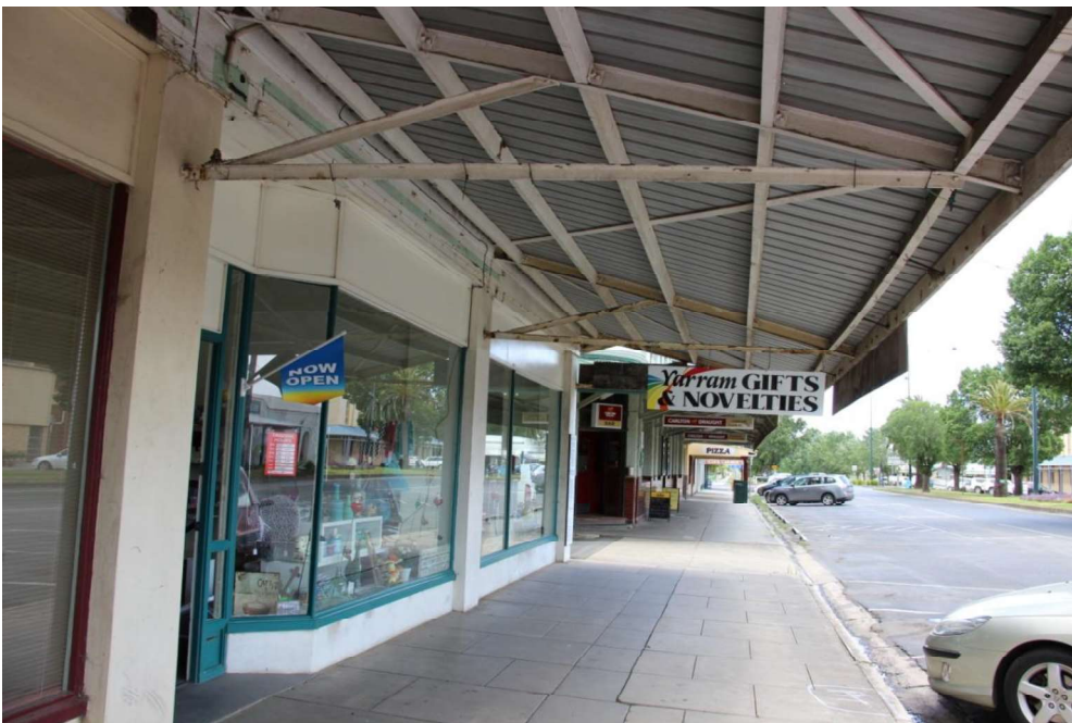
Figure D4. The shopfronts are covered by a wide cantilevered verandah with a skillion-roof (with modern cladding), which retains the original metal structure underneath. The shopfronts at ground level are early timber-framed windows with recessed entrances.
