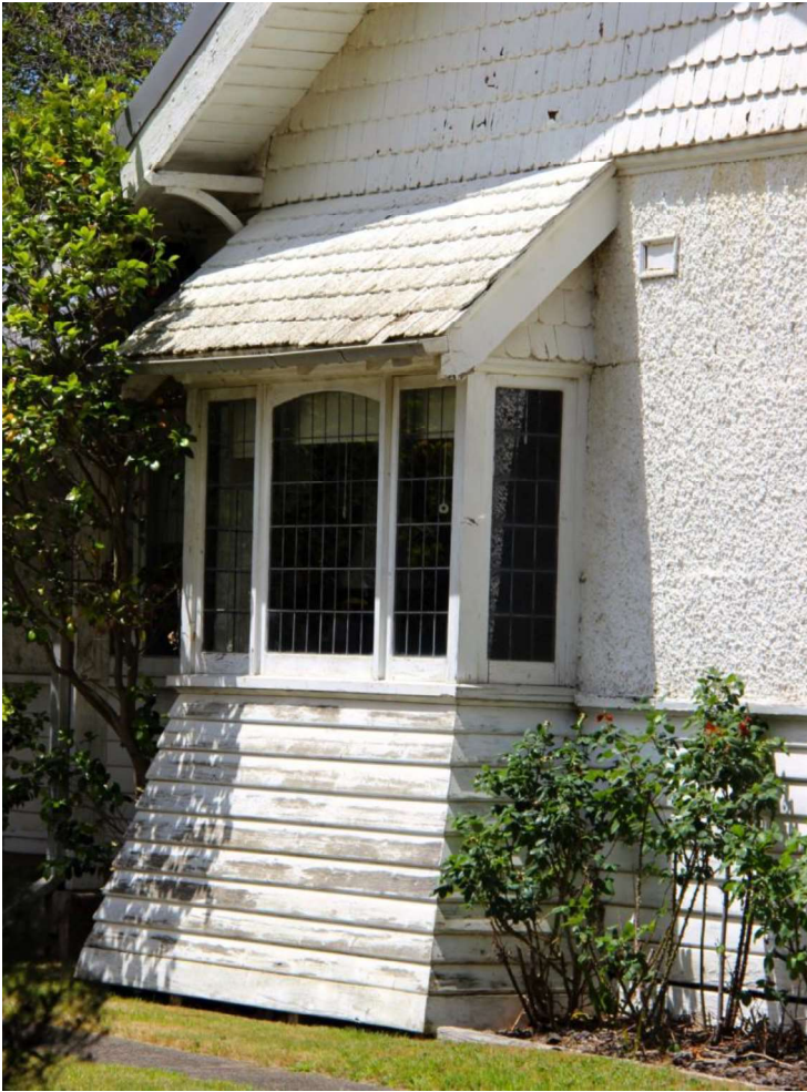
Figure D2. The projecting box window on the west elevation with a detail of the splayed base clad with mitred weatherboards, geometric leadlight timber windows and shingled roof. Half of the base of the exterior walls is timber, with roughcast render to the top half of the wall.
