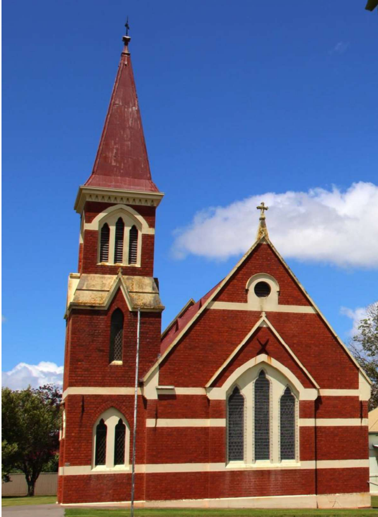
Figure D1. The church is constructed of handmade, tuck pointed red bricks, with a rendered plinth and gabled roof clad with corrugated iron. Four horizontal bands of decorative render (overpainted) run across the facade, creating dominant lines across the face-brick.
