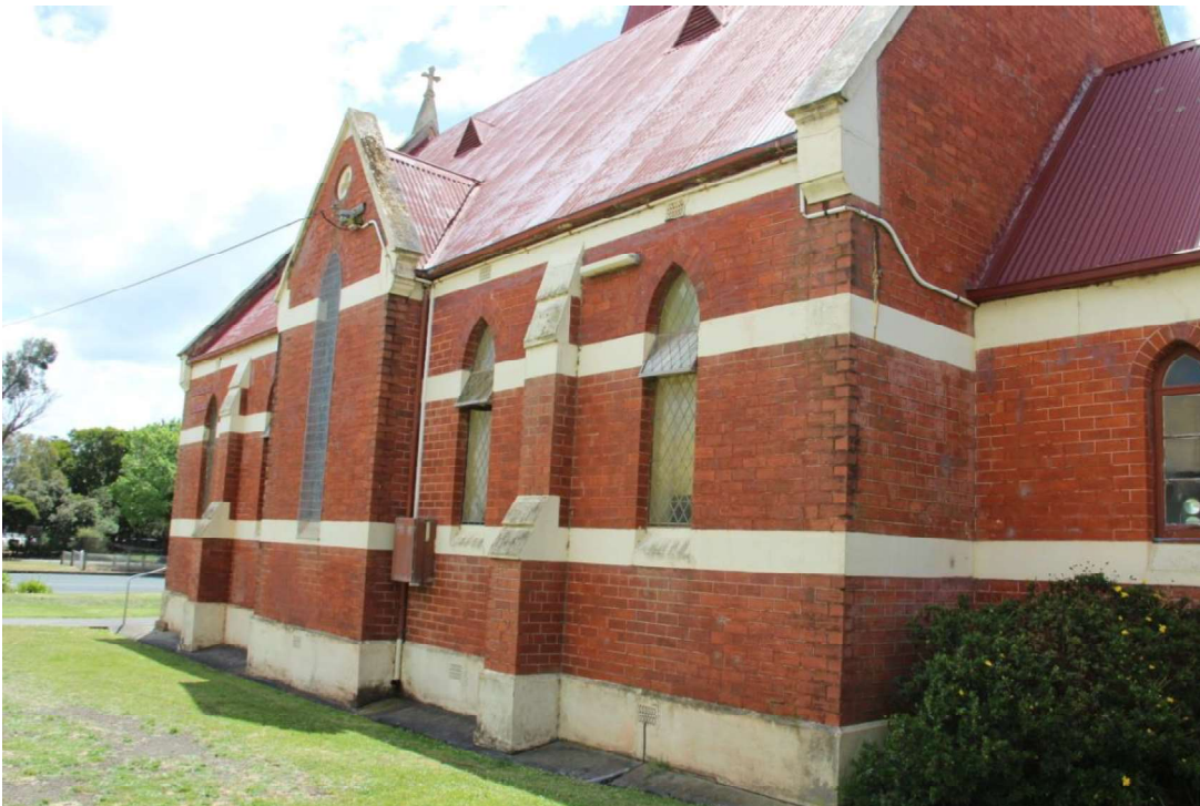
Figure D3. The south elevation. The side elevations of the nave are divided into five bays by buttresses with rendered coping. The central bay of each elevation has a (slightly projecting) gabled bay with a very tall pointed-arch window with leadlight. On both elevations, bands of decorative render (overpainted) run across the walls at sill level and impost level, (near the tops of the windows).
