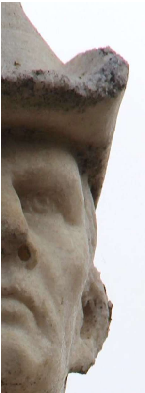
Figure D1. Detail of the damaged 'sugary' surface of the digger, particularly visible in this photos, on the edges of the hat and ears.
