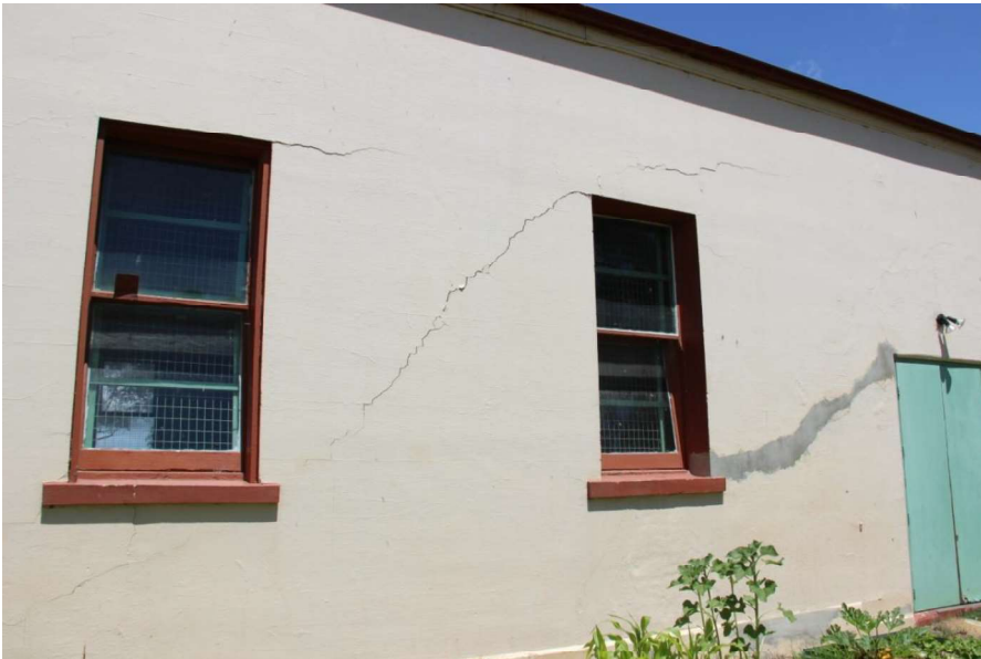
Figure D4. A detail of the windows on the north-east elevation, which are (later) timber windows. Note the cement repairs of a large crack.
