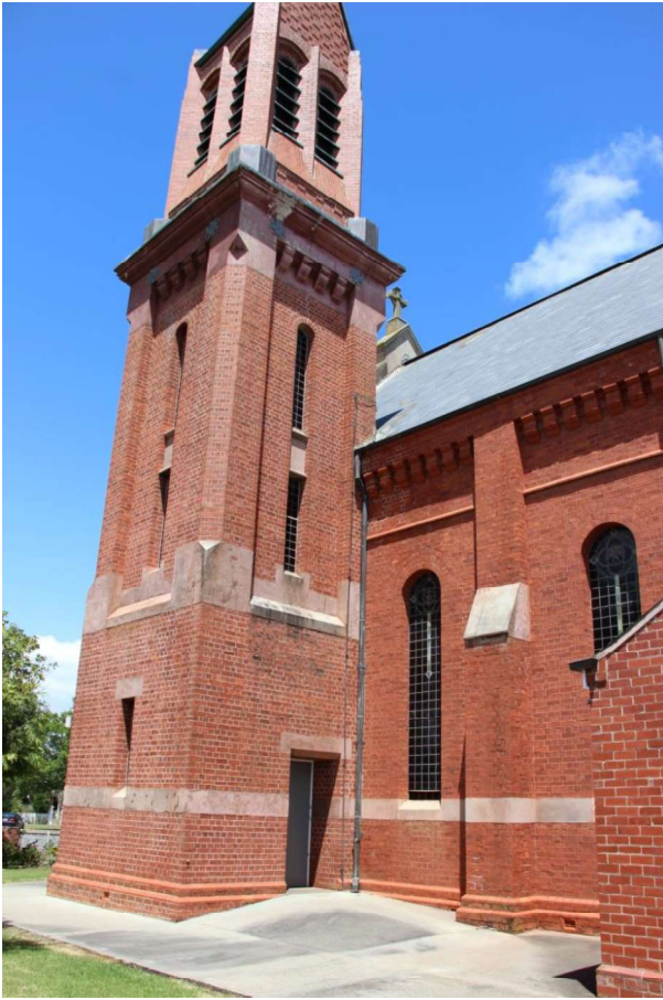
Figure D2. The gabled-roof is clad with slate, with a row of bold brackets at the eaves on the side elevations. The extent of the 1915 building comprises the five bays to the side elevations.
