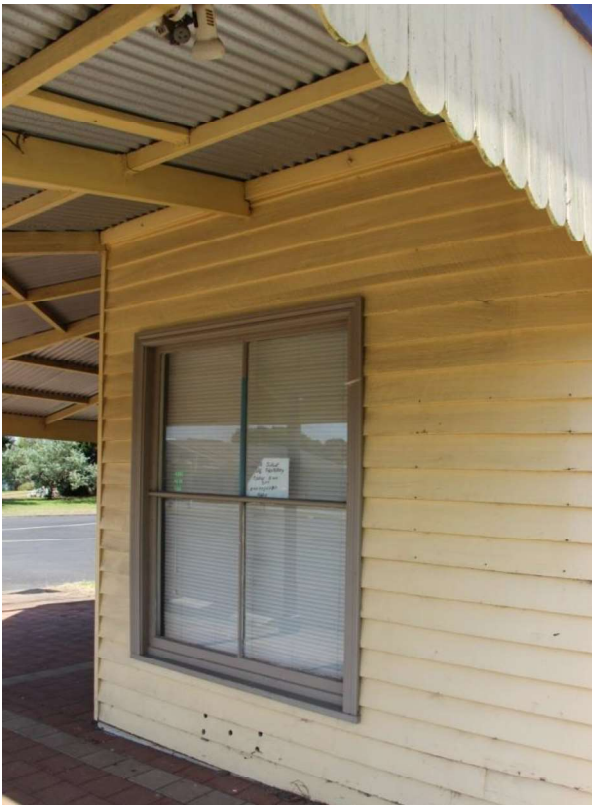
Figure D4. The two main elevations of the shopfront have large timber windows.
