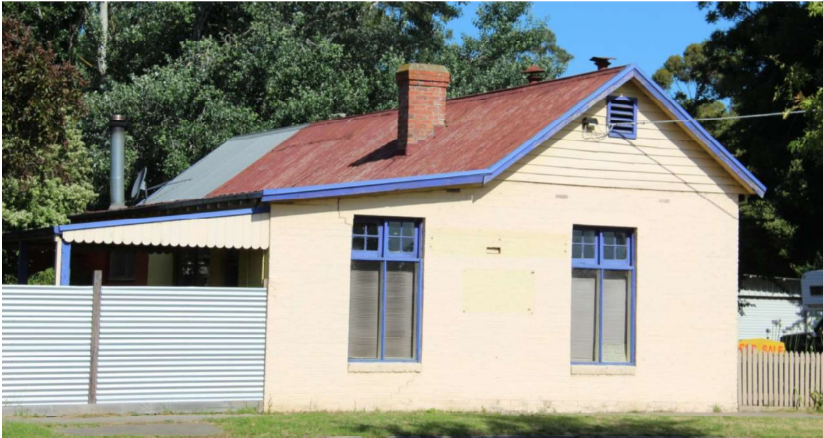
Figure D5. The north elevation of the bakery, and the east elevation fronting Tyers Street. The large brick (overpainted) bakery has a gabled roof clad in galvanized corrugated iron (painted) with round vents (c1900) to the roof, a corbelled brick chimney (unpainted) and exposed rafter ends to the eaves. The gabled end to Tyers Street is clad with weatherboards, with a rectangular vent. The lower skillion with the scalloped boarding is recent. The windows may date from c1900, but may be second hand windows inserted into this wall when the building ceased being used as a bakery.
