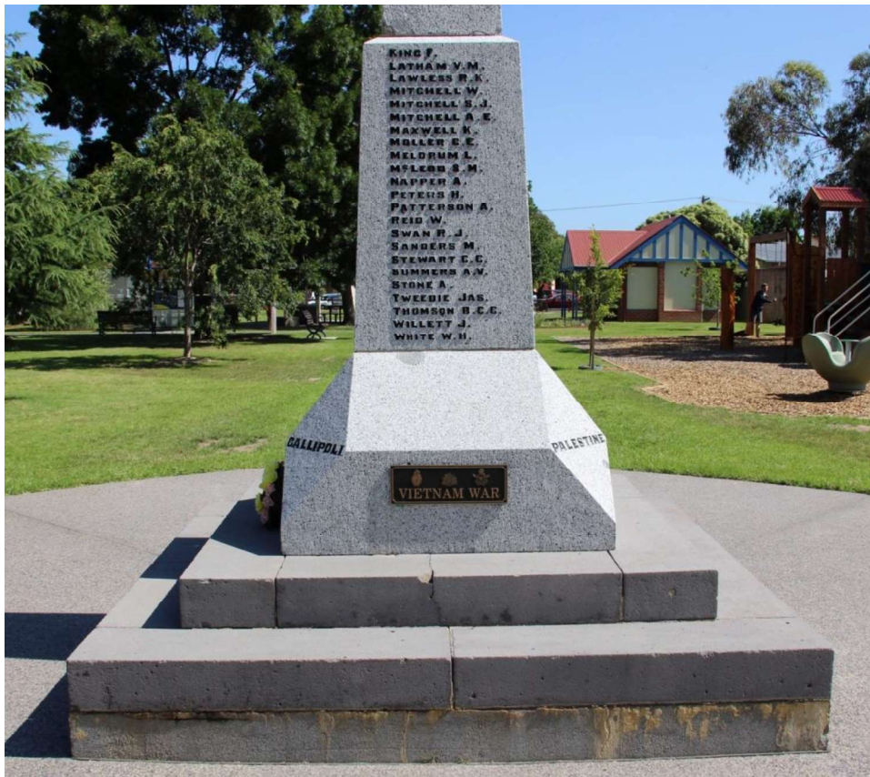
Figure D3. Detail of the concrete foundations, bluestone steps, names ( eg GALLIPOLI) incised into the granite, and names on soldiers in lead. Modern bronze and painted plaque.
