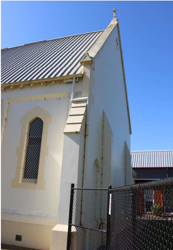
Figure D5. The rear (east) elevation has a simple treatment. It has a niche in the shape of a cross at the top of the gabled-end, like the facade, and two simple buttresses.
