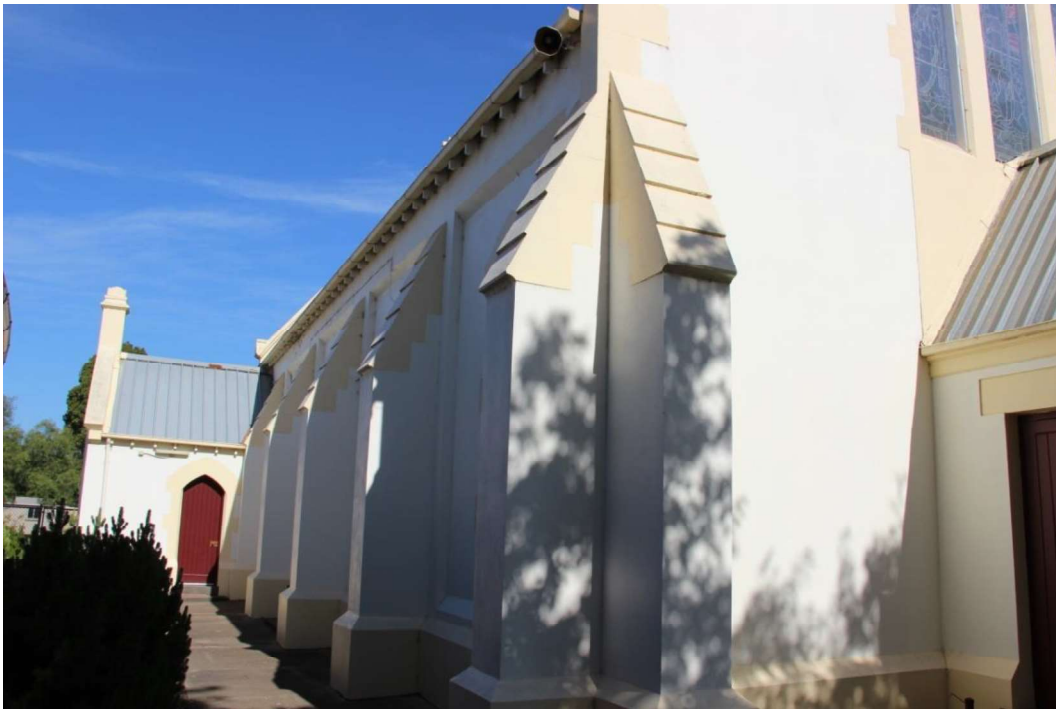
Figure D4. The north elevation has a gabled-roof vestry projecting off the chancel end, with timber ledged door (with a pointed arch opening) facing west. It has a large parapeted gable which appears to extend to form a bellcote.
