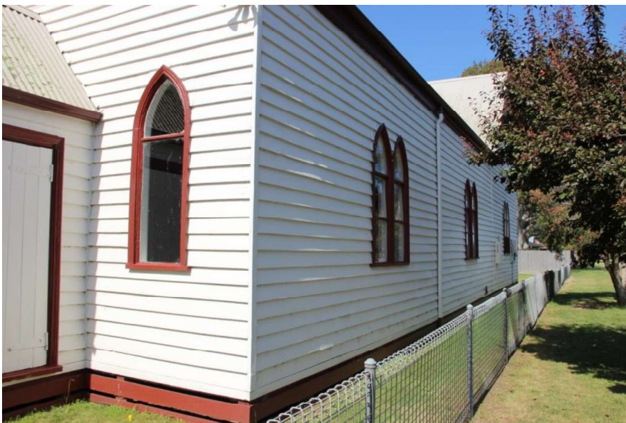
Figure D5. The south elevation of the hall has three pairs of pointed-arch windows (with clear glass) with central hoppers. There is excellent underfloor ventilation between the gaps in the base boards.
