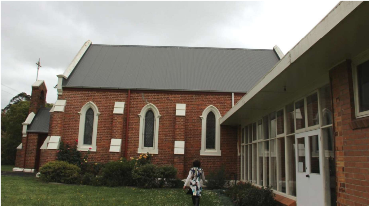
Figure D5. The east elevation. Three bays of the east elevation are visible. The c1960s cream brick addition adjoins the church in the fourth bay, at the rear of the church.
