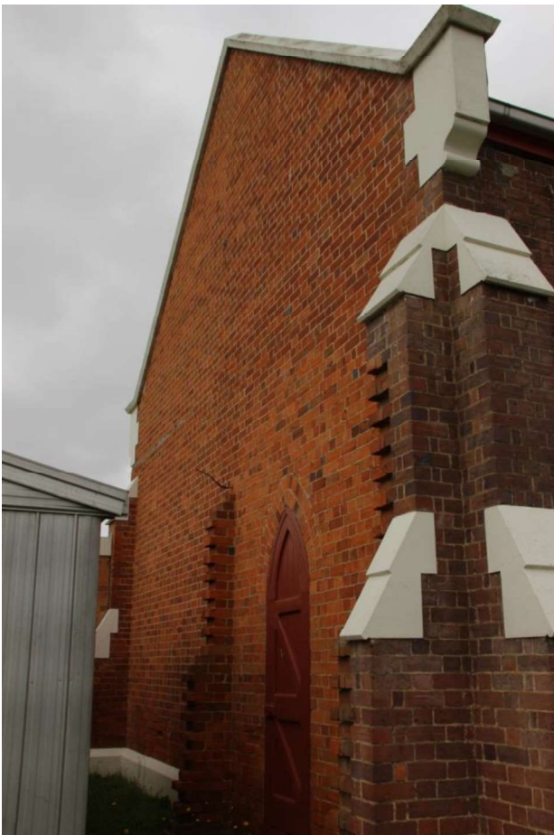
Figure D6. The rear (north) elevation is of red brick. Keyed bricks remain on the right side, that were ready for an extensions that never eventuated. The space in between the keyed bricks has a pointed-arch opening with a timber ledged and framed door.
