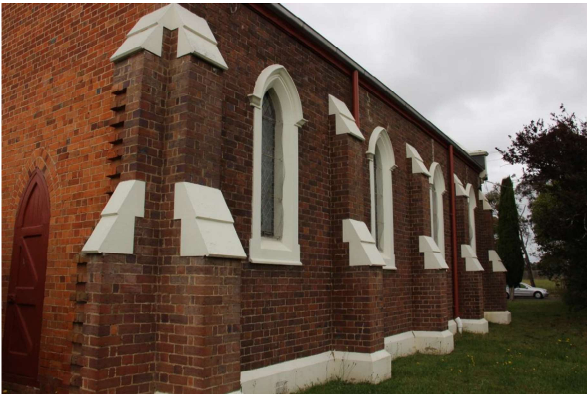
Figure D4. The west elevation. The side elevations are broken into four bays but buttresses, each bay with a single window like those of the façade.
