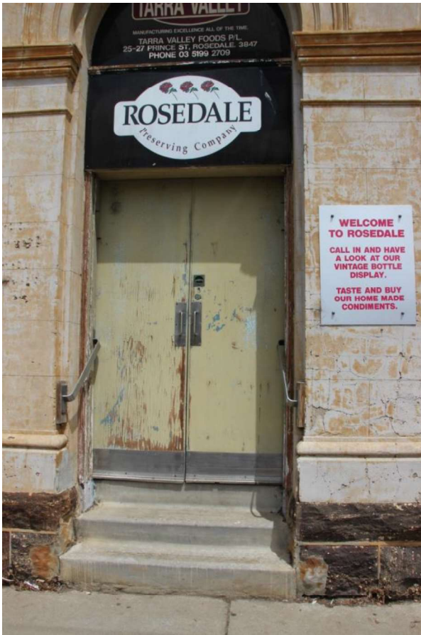
Figure D5. A detail of the facade and entrance showing the unpainted original local stone plinth ruled lines to the unpainted rendered wall planes, and the later doors, metal balustrades and concrete steps.
