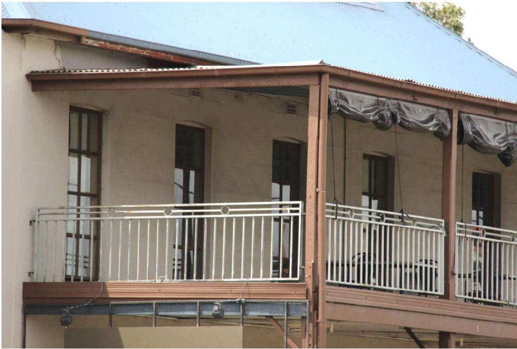
Figure D2. The tall openings to the first floor of the south elevation are all original (with modern multi-paned windows that replaced the original French doors).
