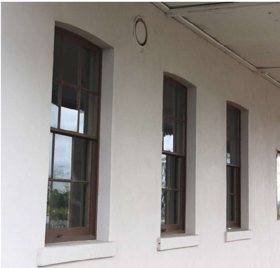
Figure D3. The ground level retains three original six-over-six sash windows on the southern elevation. All openings to the south elevation have radiating voussoirs above, and the windows have projecting sills (all rendered and overpainted).
