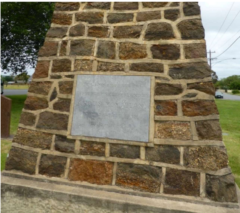
Figure D4. Detail of the 1927 Angus McMillan cairn, showing the local stone blocks, heavy protruding lime- mortar joints, 'concrete' plinth and marble plaque with hand cut incised lettering.
