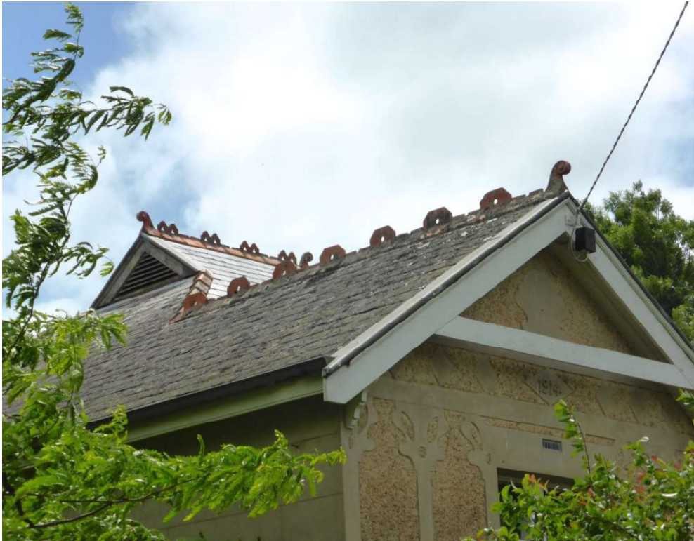
Figure D3. The elaborate hipped and gable roof is clad in slates, with terracotta ridge crests and finials. The decorative wall pattern can be seen in the gable end.
