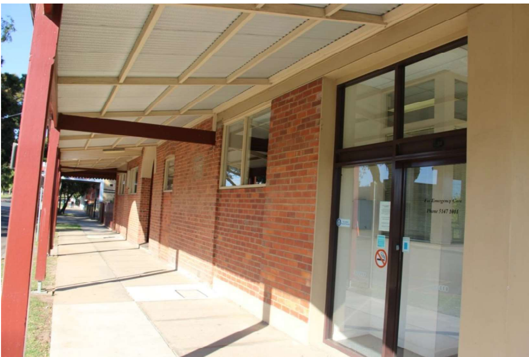
Figure D5. The ground floor on the west elevation retains part of the original external wall. Modern windows and doors have been inserted (in 1975). Small high-set windows have been inserted, in some cases in original openings (with the remainder of the opening bricked up).
