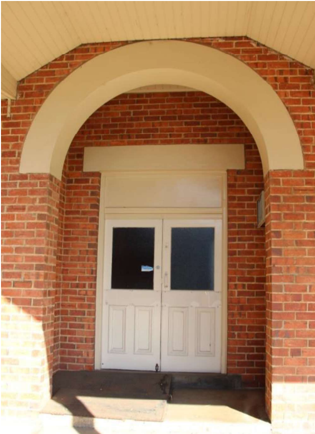
Figure D4. The ground floor retains the original recessed entrance, entered by a semi-circular (rendered) arch. The ceiling of the recessed porch is timber-lined.
