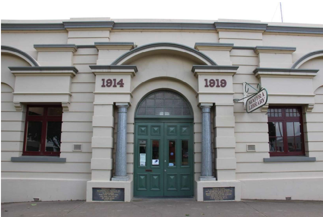
Figure D3. The elaborate entrance with the foundation and memorial stones and pair of polished granite columns with Tuscan capitals, which support the entablature which bear the dates '1914' and '1919'.
