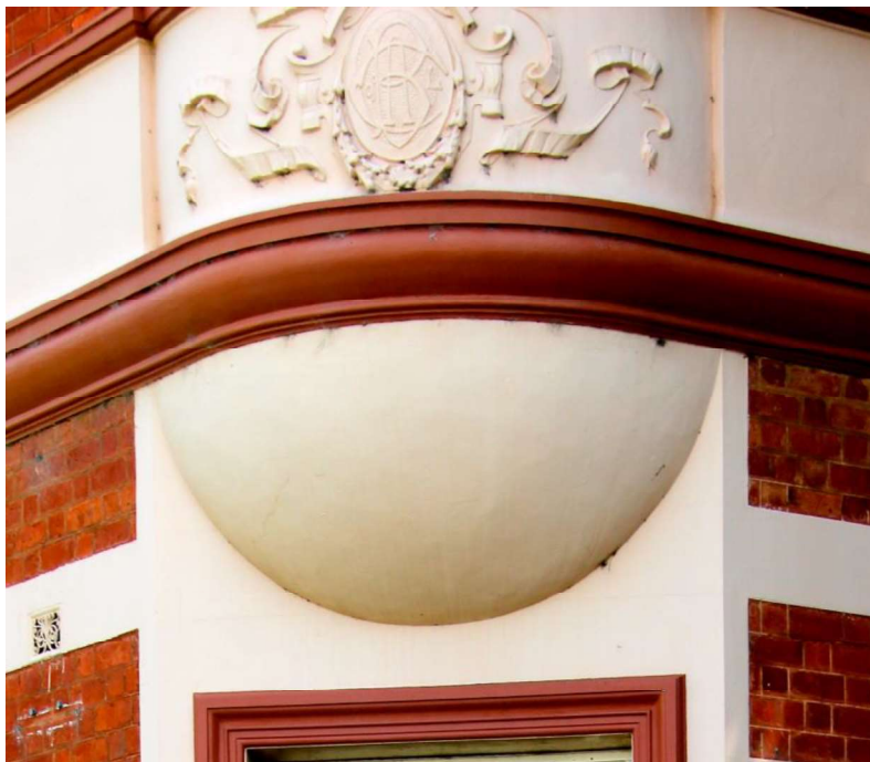
Figure D4. Detail showing the oriel balcony, rendered moulding, flat rendered bands, bank insignia in relief render, decorative wall vent and tuckpointed red brickwork. All the render on this building was originally unpainted and remained that way for about 80 years.
