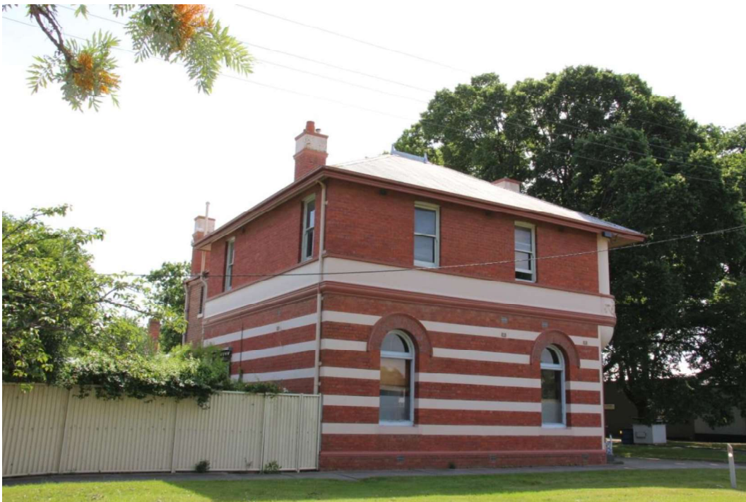
Figure D2. The north-west and south-west elevations. The chimneys are consistent in style on the front and rear portions of the building.
