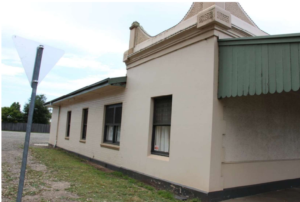
Figure D5. The 1922 facade continues on the west elevation to the width of one bay, where the parapet is again accentuated above. The post-1939 brick addition extends to the north.
