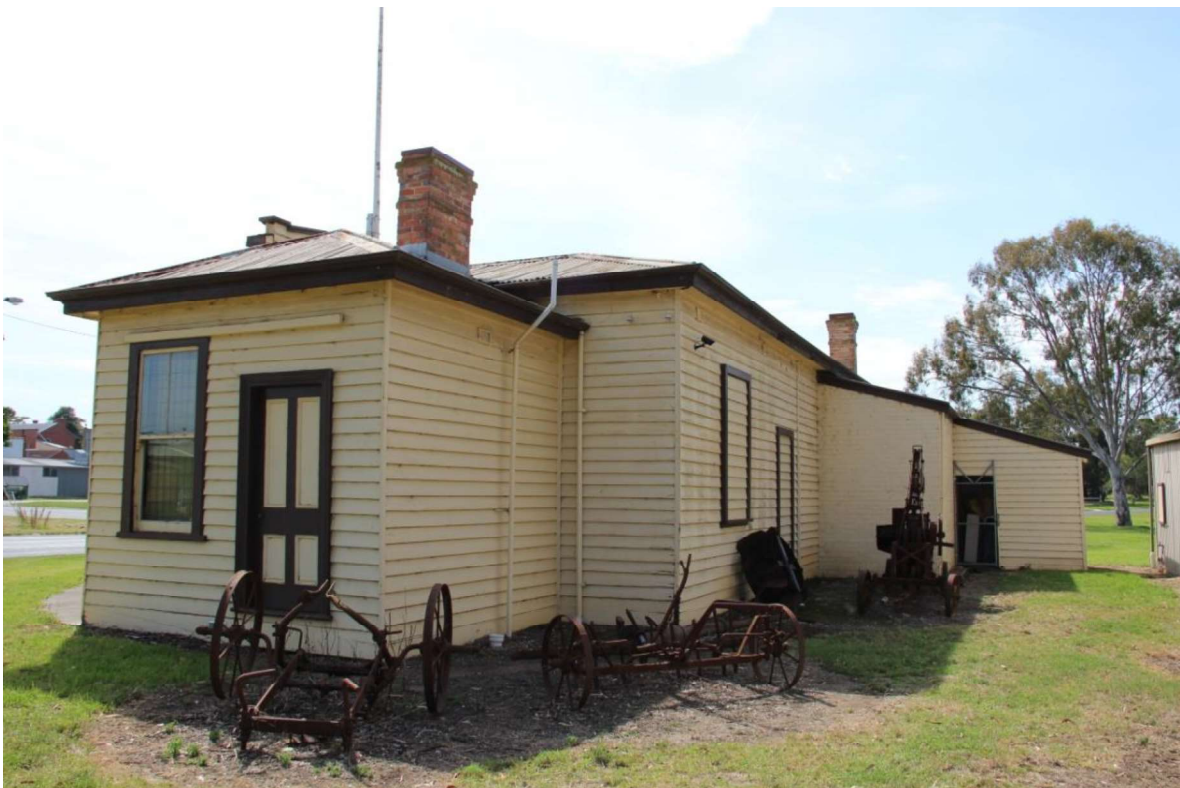
Figure D3. The north-west elevation with its original timber door and window, with the verandah removed. The rear elevation has two openings that have been in-filled with weatherboard, and two later additions to the rear.
