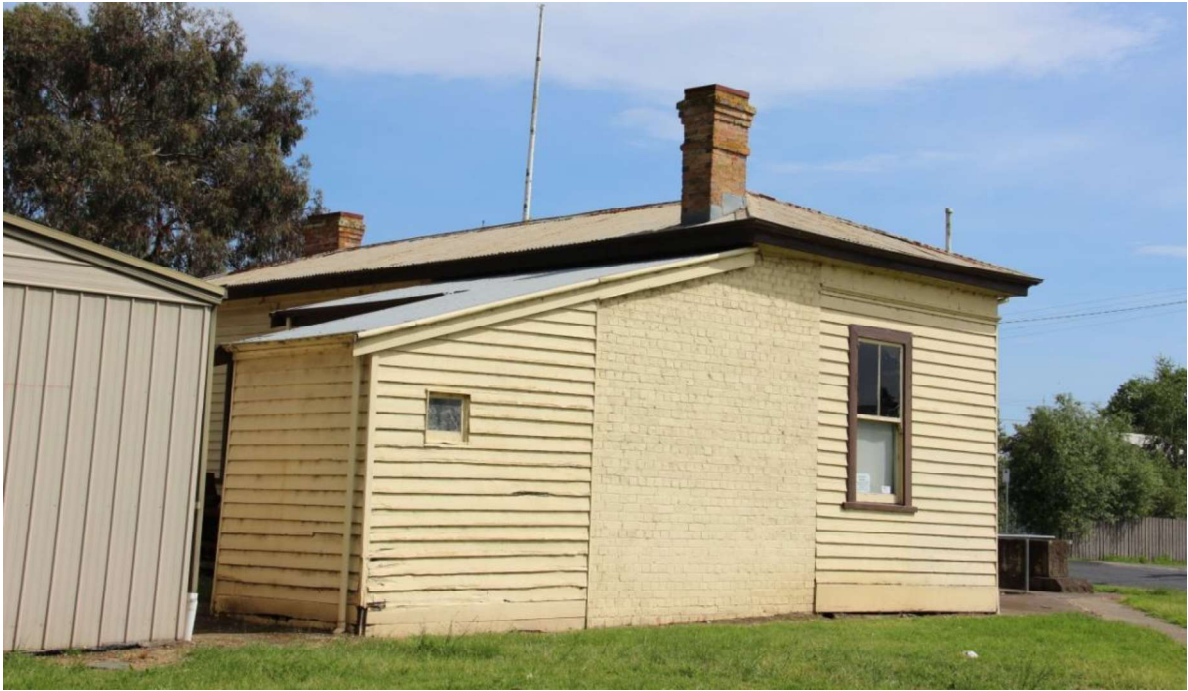
Figure D4. The south-east elevation, showing the two later additions with a skillion-profile roof. The brick section appears to form part of the chimney (reconstructed after its relocation in 1975).
