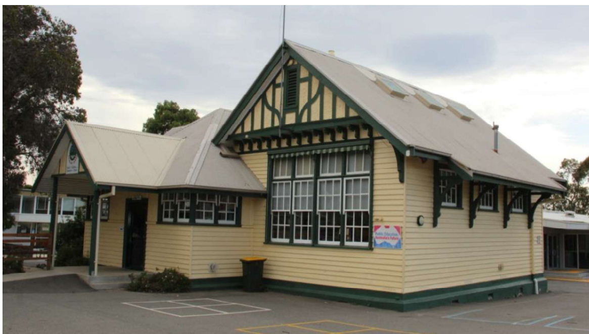
Figure D6. The front (east) elevation faces Temple Street. The weatherboard building has an asymmetrical plan and a complex hip-and-gabled roof recently clad with Colourbond. The wide timber-lined eaves are supported by large ornate timber brackets. The multiple gabled ends have a flying gable with roughcast render and timber strapping (with curvilinear details) to the gabled
