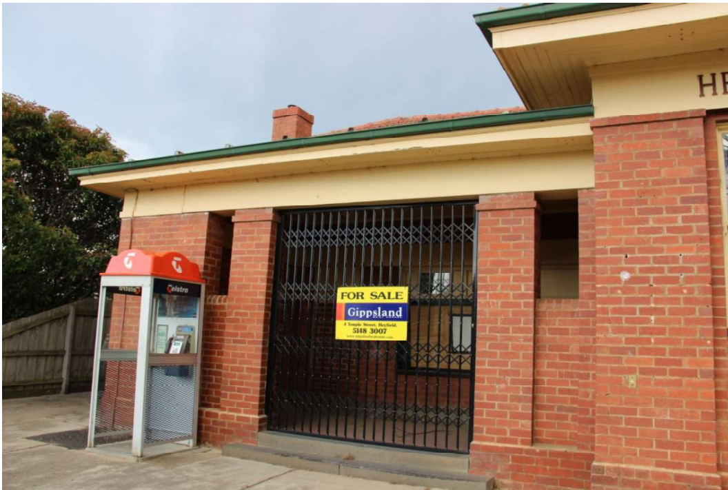
Figure D3. The entrance porch to the left of the facade, which is under a separate roofline.
