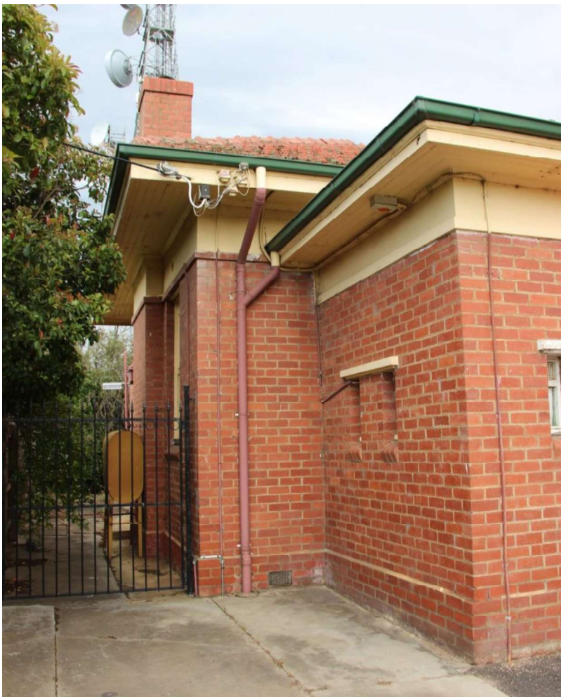
Figure D4. The chimney stack stands on the exterior of the elevation. Three small windows are
