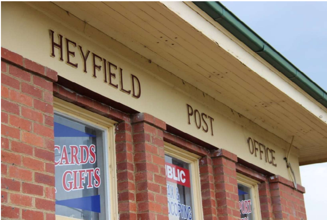
Figure D2. The wide eaves which are timber lined, and the name of the post office on the smooth band of decorative render.
