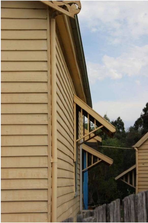
Figure D3. The west elevation has openings covered by c1990s window hoods.
