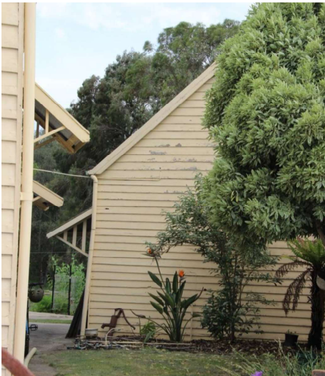
Figure D4. The long weatherboard building to the rear of the house, with a steeply pitched gabled-roof (probably the original police stables; it is evident in the 1890s photo, Figure H1).
