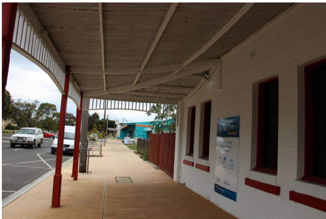
Figure D3. The openings to the north and west elevations appear to be very similar to the Victorian era openings, in the Victorian facades (see Figures H1 & H2). Note the concave verandah structure.
