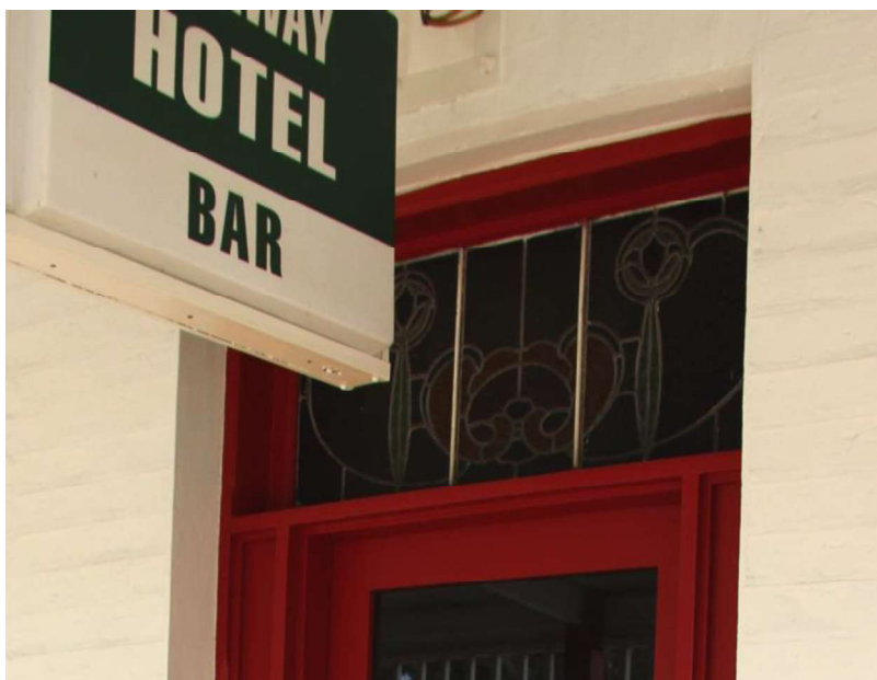
Figure D4. The corner entrance retains leadlight highlights with an Art Nouveau influence dating from the c1918 construction.
