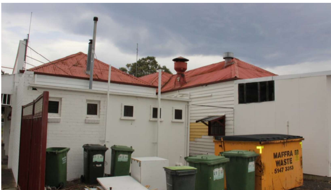
Figure D5. The rear (south) elevations, dating to the Victorian period, are clad in weatherboard, with the hipped roofs evident above.
