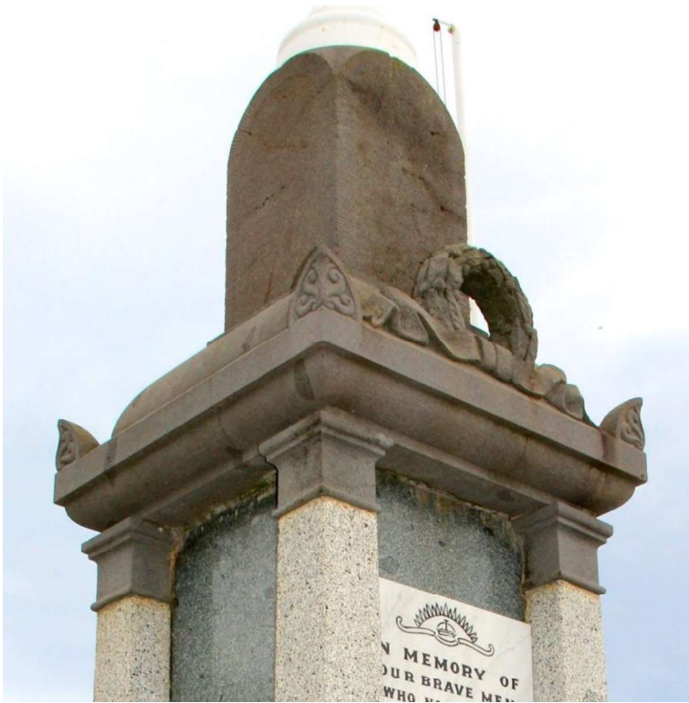
Figure D3. Detail of the top of the cenotaph showing finely tooled bluestone, polished Harcourt granite piers and Orbest granite panels, with some water damage occurring at the top of the panels.
