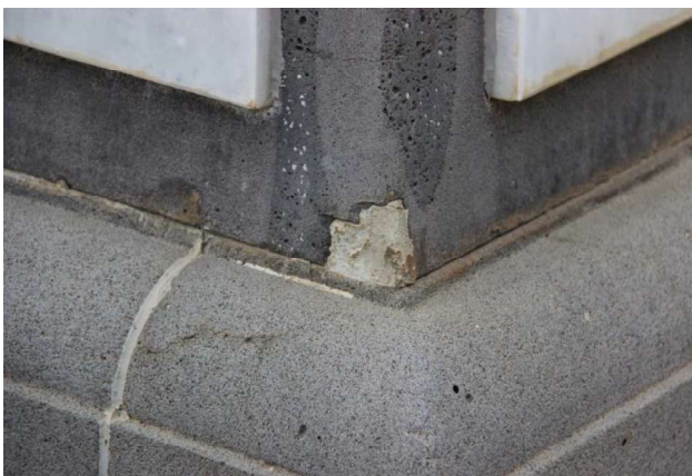
Figure D2. Detail of damaging repairs using a 'plastic type' substance in the joints instead of
