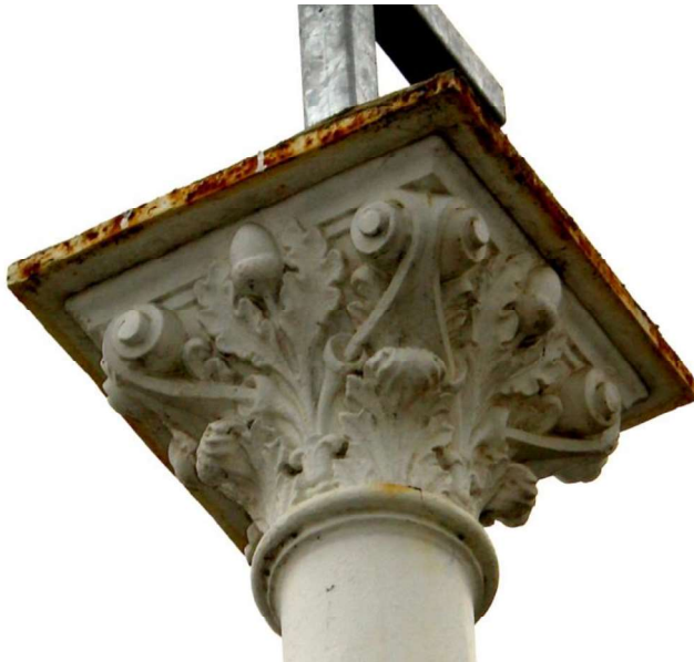
Figure D4. Detail of white painted rusting cast iron column with recent metal cross above.
