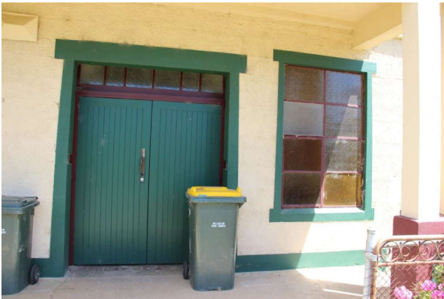
Figure D2. Underneath the porch is an entrance with a pair of wide timber ledged and framed doors with a multipaned metal-framed highlight. The door has a rendered lintel and sides (overpainted); the render to the sides tapers to the tops, giving an Egyptian nuance to the entrance. To the right is a metal-framed 8-paned window of yellow pressed glass, with a rendered sill, lintel and sides, forming a frame to the window.
