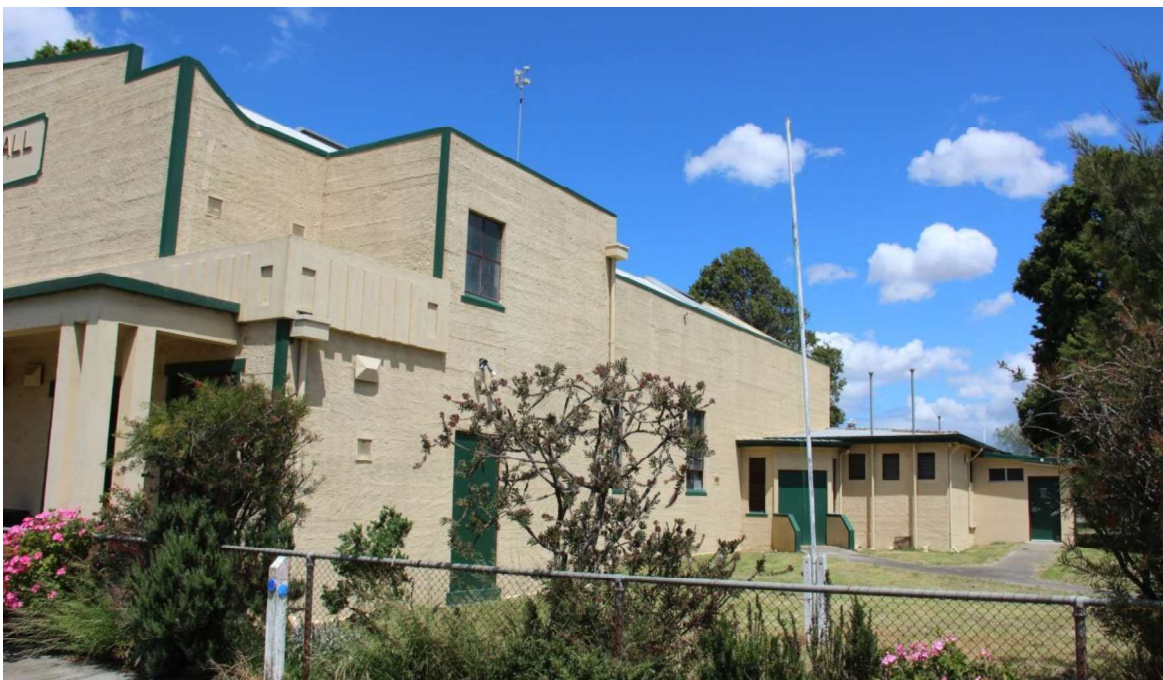
Figure D4. The west elevation has a timber ledged and framed door at the north end and 4 and 8-paned metal-framed windows with rendered sills. A large single-storey addition is constructed off the rear (south) and west elevation of the hall, which serves as the toilets.
