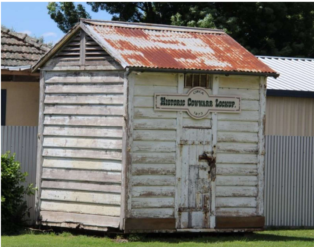
Figure D3. The small iron cage lockup with its gabled roof, half-round spouting and weatherboard wall cladding. It retains timber vents at the gable ends, a metal grill above the door, and its original (or an early) door with full-width hinges and a number of early locks.
