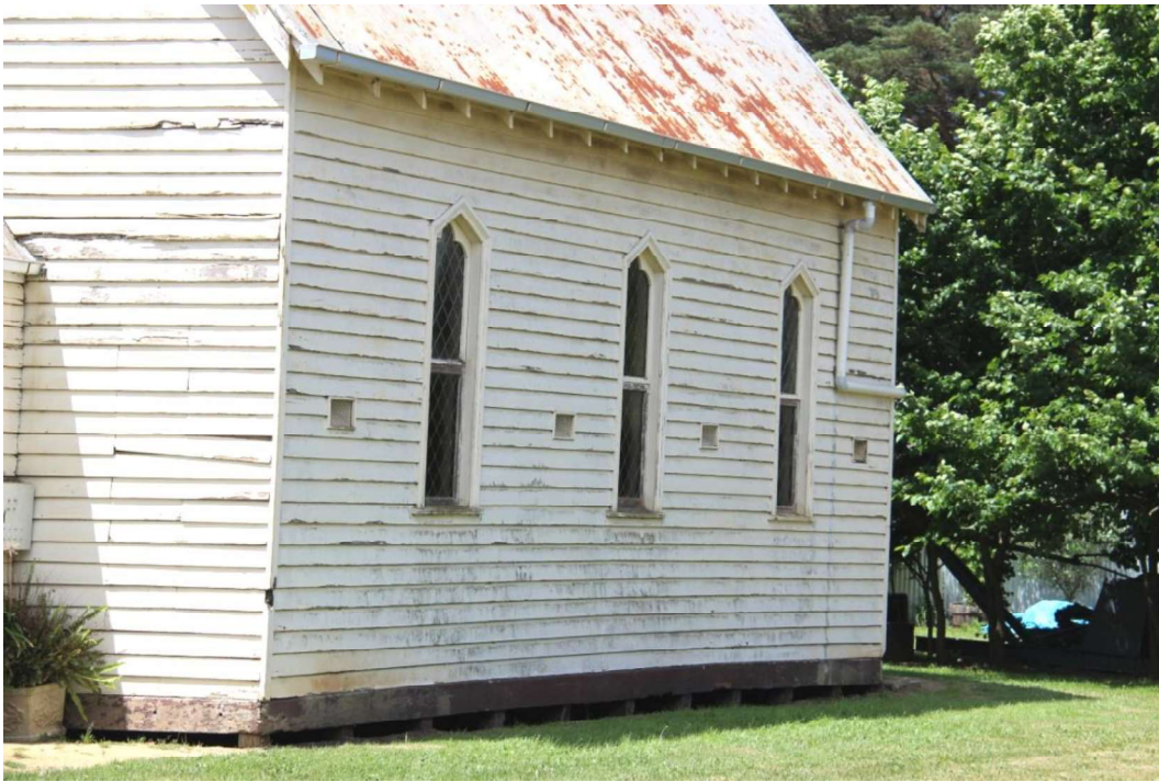
Figure D2. The south elevation with the three leadlight windows in a diaper pattern and trefoil motif to the top, set within the pointed-arched timber frame.
