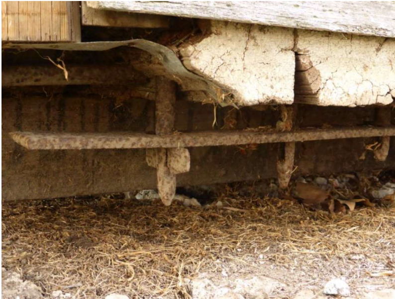
Figure D4. The lock up is constructed of an iron cage clad in timber, making it suitable for prefabrication and easily transported. The ends of the iron rods can be seen at the level below the door.
