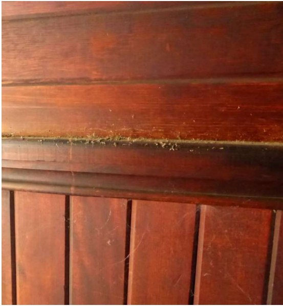
Figure D2b. Interior showing a detail of the carpentry of the red pine timber lined walls and dado.
