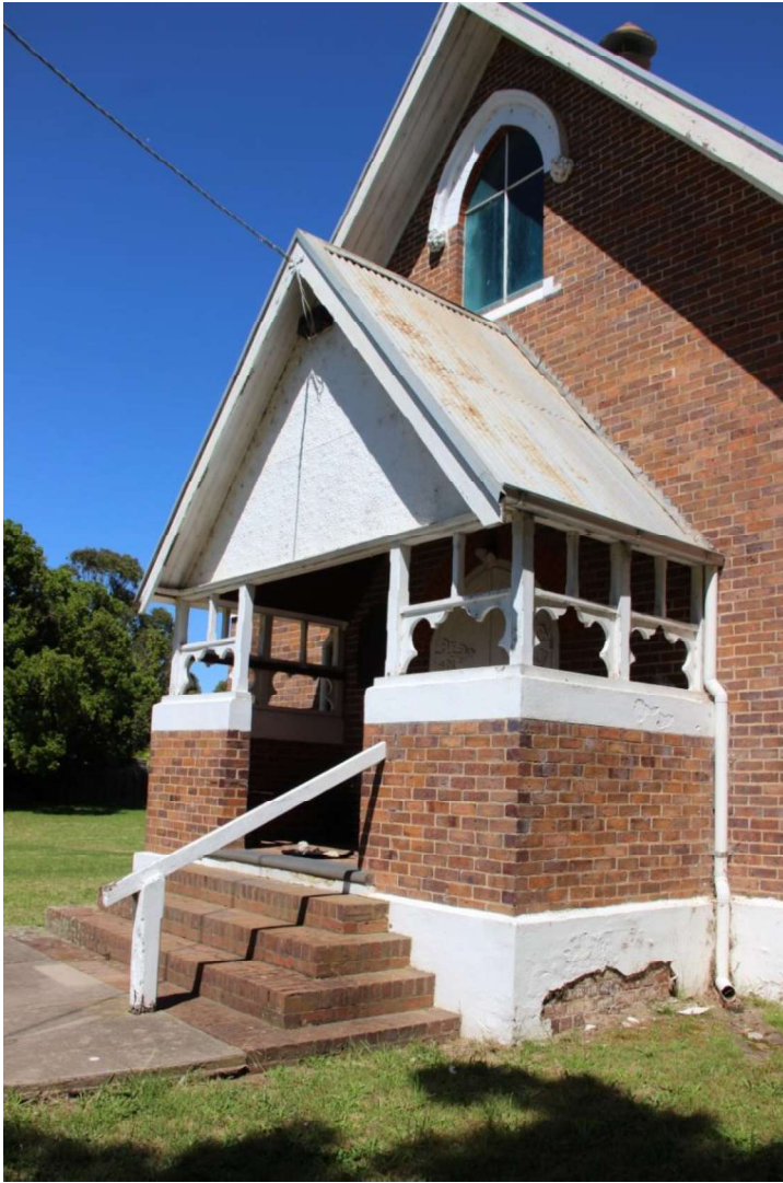
Figure D2. The entrance porch with the pressed metal cladding to the gabled end imitating a rough-cast render, timber tracery and brick balustrade. Note the damp damage to the render of the plinth.
