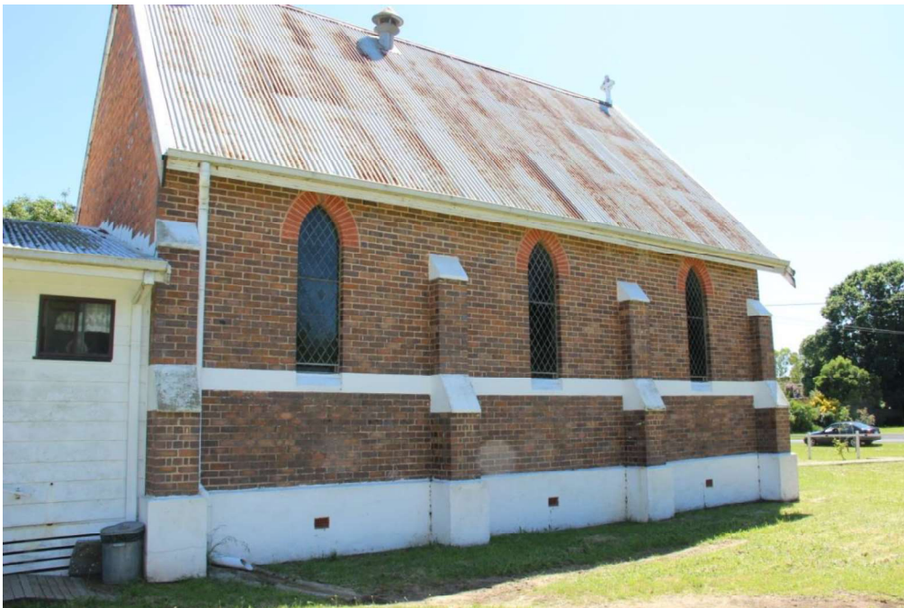
Figure D4. The side elevations of the 1908 brick church are divided into three bays by four buttresses with rendered coping. Pointed-arch windows have diaper-pattern leadlight of coloured glass, with red-brick voussoirs above. Note the lapped galvanised corrugated iron roof with original ventilators.
