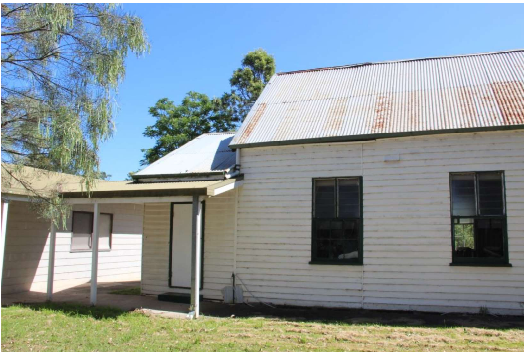
Figure D5. The rear section of the southern elevation. The modern weatherboard building to the rear of the 1874 church is connected to the smaller weatherboard room attached to the rear of the church by a modern breezeway that covers an entrance to the church off the southern elevation.
