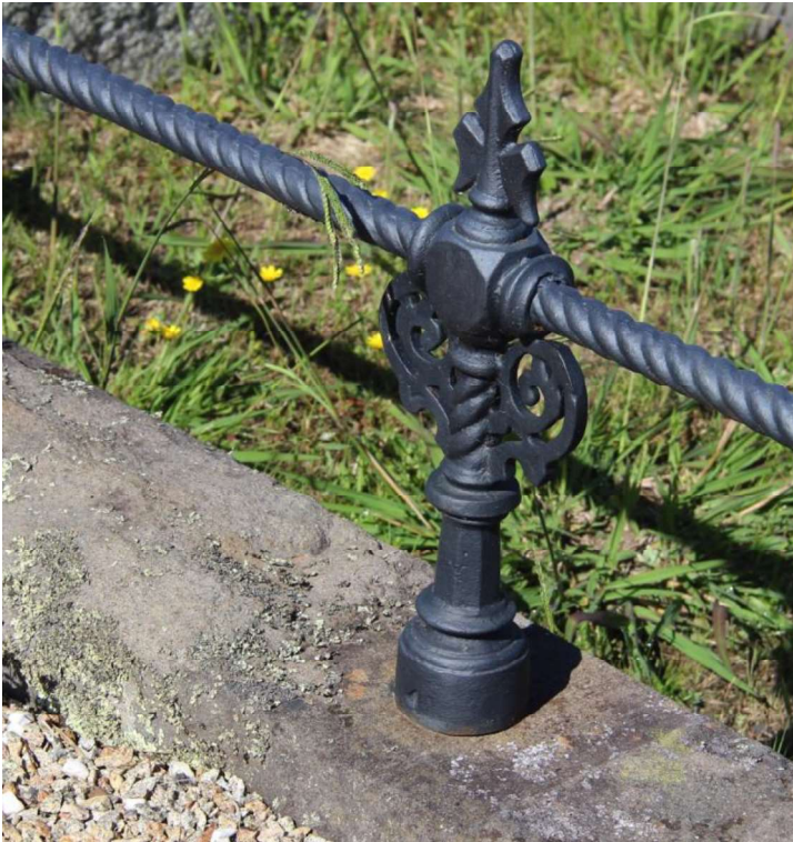
Figure D4. Detail showing lichen on the bluestone plinth, and 'restored' cast iron rail and post.
