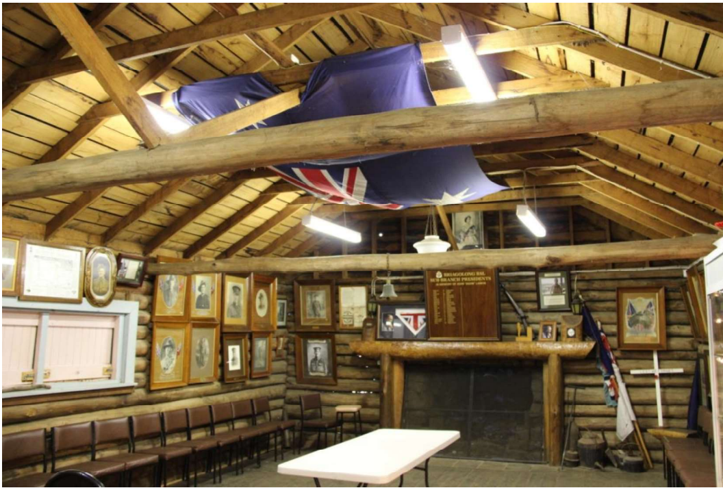
Figure D5. The interior of the log cabin is in very good condition and has a very high level of integrity, retaining its original timber elements. The interior walls are not lined, with the Yellow Stringybark logs evident.
