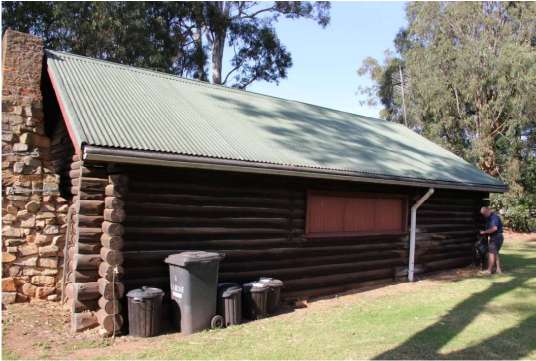
Figure D3. The north elevation with its wide timber-framed window with its original timber shutters (like the main elevation).
