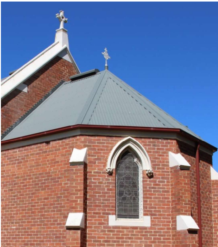
Figure D4. The windows to the bay at the chancel end have ornate leadlight.
