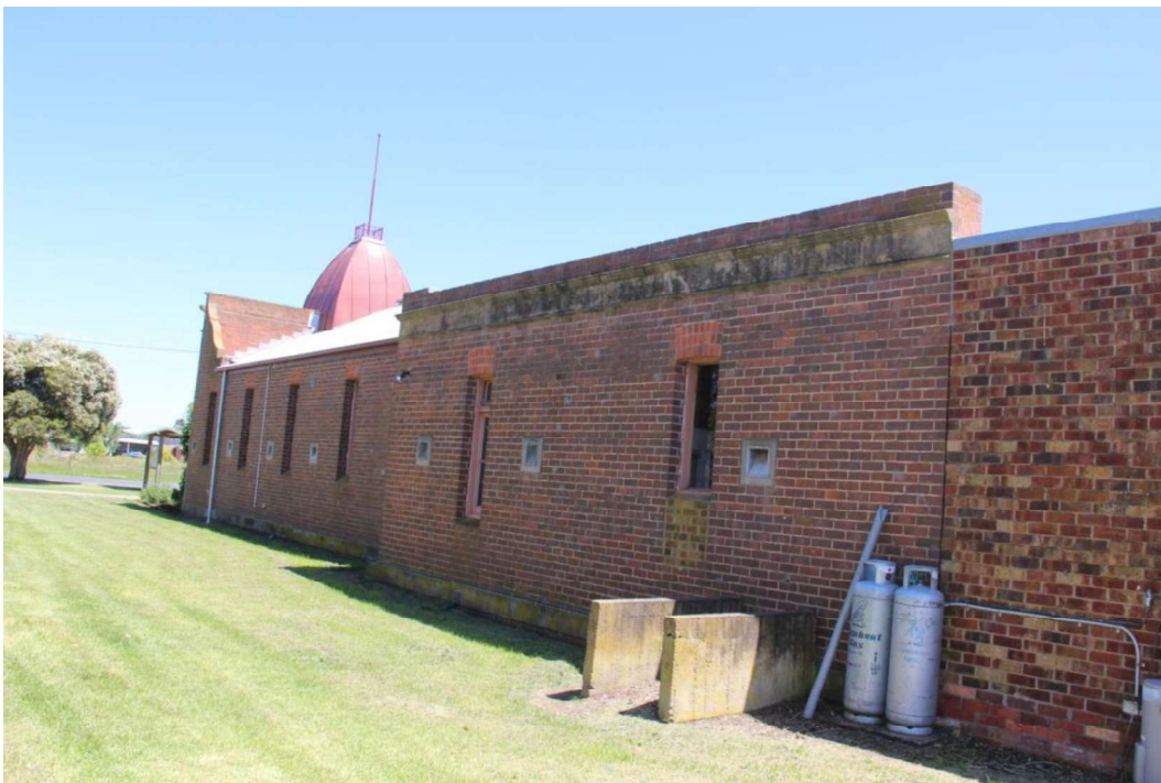
Figure D4. The south elevation showing the rear of the parapet which continues onto the side elevations. The windows have the same treatment as those on the facade. The rear section of the 1904 building has a parapet with a band of roughcast render.
