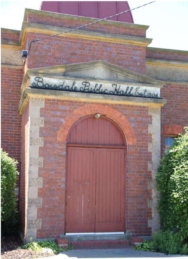
Figure D3. A detail of the original tuck pointed English bond entrance porch with its arched entrance, pediment, rendered dressings and metallic glazed bricks.
