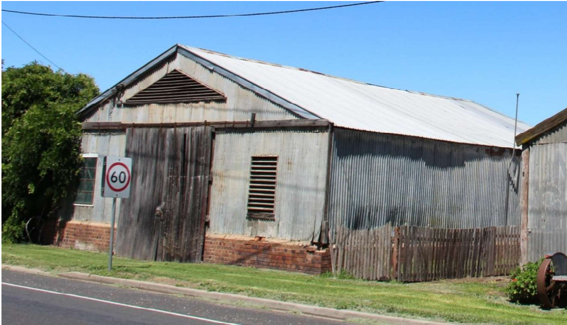
Figure D3. The blacksmiths and wheelwrights building at 37 Main Street. The gabled roof building retains its original sliding timber door, galvanised iron cladding and brick plinth and some timbered louvered openings.
