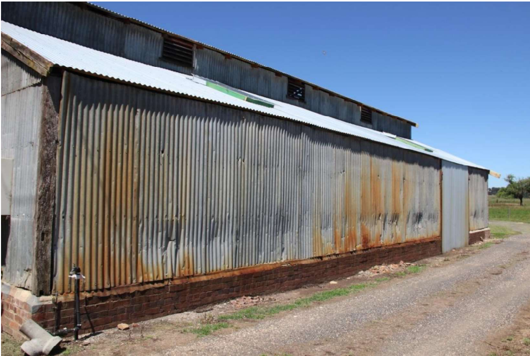
Figure D2. The northern elevation of the stables, with the galvanised corrugated iron walls sitting on the brick plinth, the timber-louvered vents to the clerestory level, and modern skylights to the roof planes below. One large opening is located on this side elevation.
