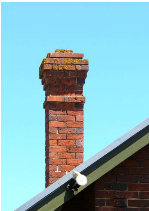
Figure D6. Detail of the corbelled chimney made of the bricks from the Foster family kiln. The bricks and chimneys on other Foster sponsored homes in Boisdale are very similar.
