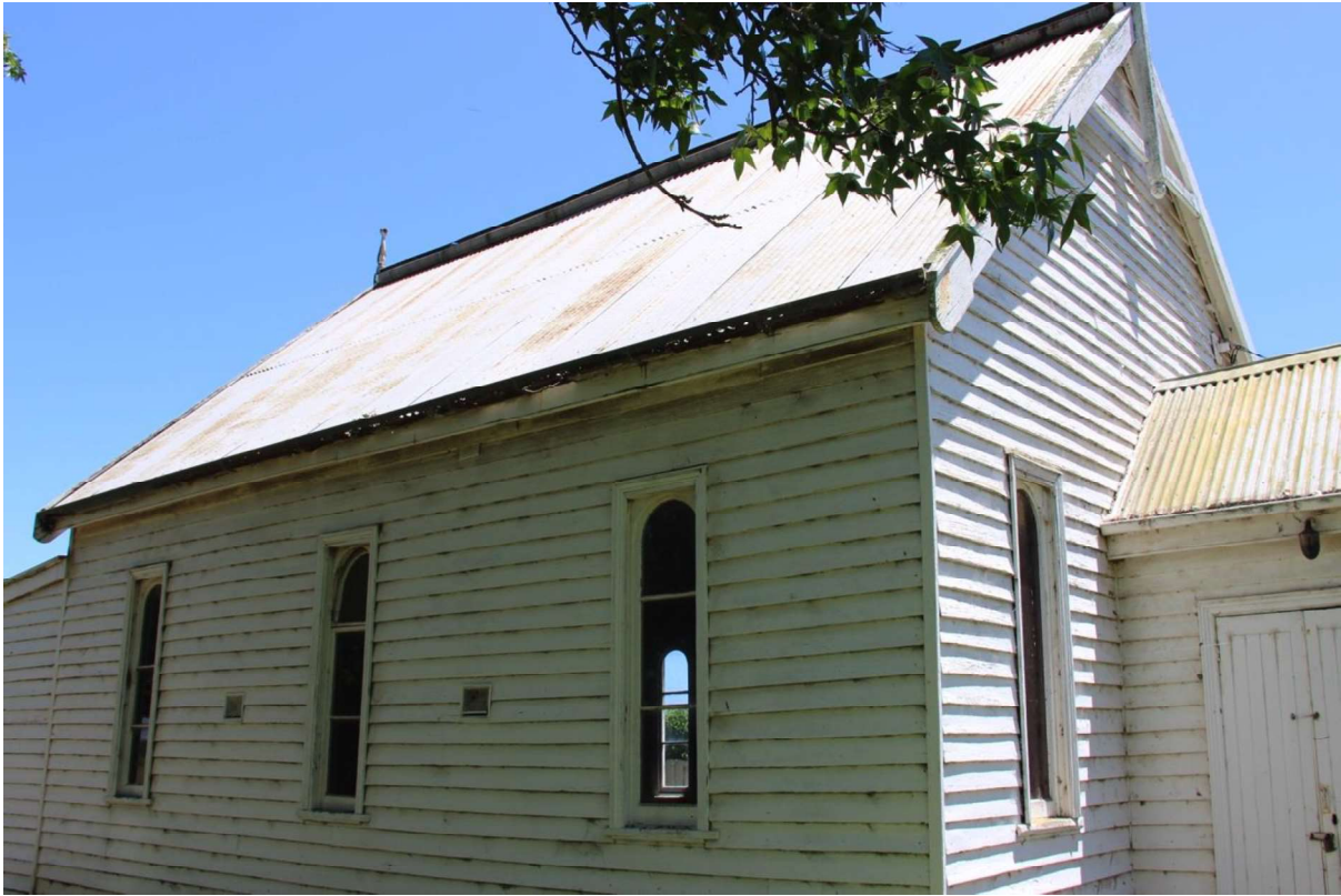
Figure D3. The side elevations comprise three tall windows, with small vents in-between. The windows to the nave have clear glass in three parts; the top portion being a hopper window. The central window has an open hopper in the photo above (not all windows are original). To the rear of the church is the later skillioned-roof addition which is not significant.
