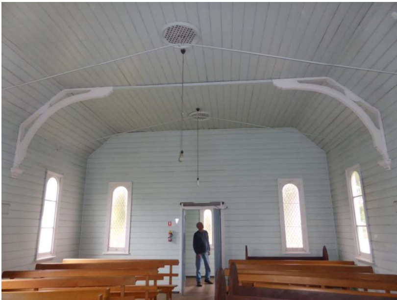
Figure D4. The timber-lined interior of the church with its covered ceiling, metal trusses, decorative metal ceiling vents and decorative timber trusses. (BHG).
