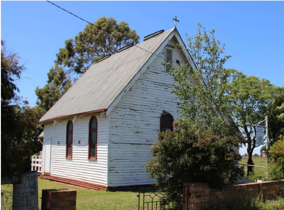
Figure D1. The weatherboard nave has a steep-pitched gabled roof clad in corrugated iron and semicircular-arched windows with coloured leadlight.
