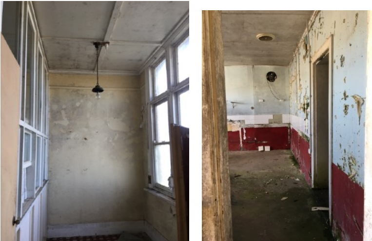
Figure D13. Area D. Typical views of the asbestos clad ceiling and walls of the interior of the 1931 offices.
