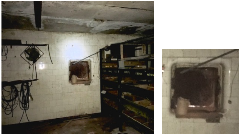
Figure D7. Area B. Note the white glazed tiles on the walls, red-brown hexagon tiles on the floor and concrete roof and detail of hatch which opens out to the front (south elevation) of the building.
