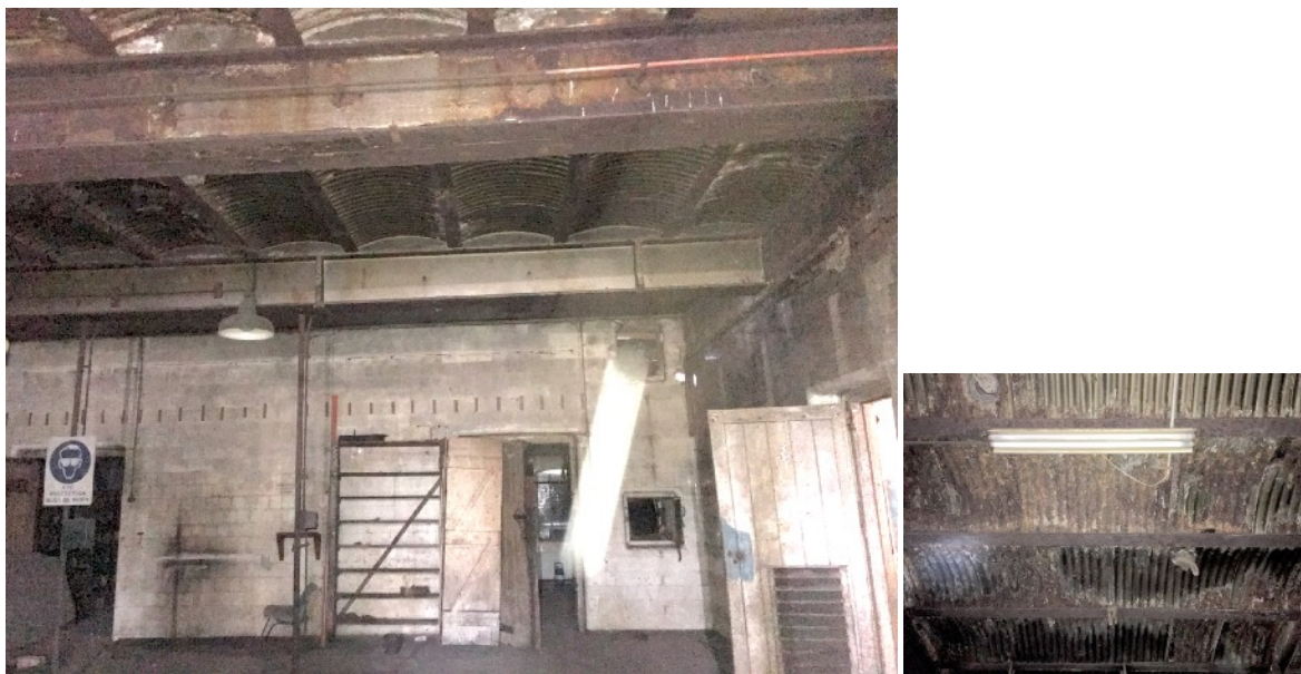
Figure D5. Blue Area A. View looking south towards the doorways into Areas B and C. The door on the right goes into Area F. Note all the walls are lined with glazed white tiles (now dirty) as are the architraves and reveals, the floor is lined with matt finish hexagon shaped brown-red tiles and the ceiling appears to be comprised of wrought iron joists supporting arched, deep-gauge (?) corrugated iron. The roof appears to be supporting a concrete floor. The method of construction is now rare, and appears to be similar to that used in the Queens Warehouse, Melbourne and described by Miles Lewis as 'Lysaght's Galvanized Tinned Iron 20 Gauge [sic]'; 'Heavy Weight ... equal to sample'; and 'Traegerwellblech'. "In 1902 Lysaght's Metal Trades Referee listed 'weight-bearing' Lysaght Orb iron of four inch [102 mm] pitch and 2\frac{1}{2} inch [38 mm] depth." (Structural Corrugation: February 2017 8.05.29. The roof was most likely used in this case to assist with keeping the building cool. It is also noted that the girders and corrugated iron are corroding. It is recommended that a forensic and heritage structural engineer investigate the actual method of structure and recommendations for repair.
