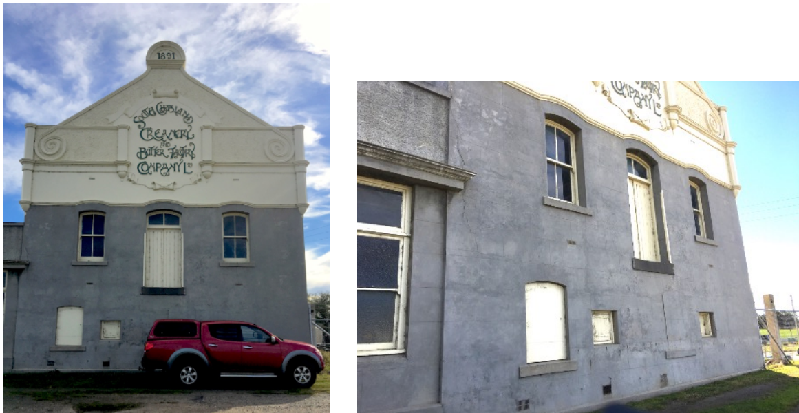
Figure D1. Blue Areas A, B, C, H, I, J. The 1908-9 former Yarram Butter Factory building south (front) elevation. The 1891 date refers to the date the Yarram Dairy Company commenced, not the date of this building. The front facade has a high degree of integrity as a fine example of the Federation Anglo-Dutch style applied to an industrial building. The original tuck pointed red brick walls (now rendered) contrasting with the elaborate rendered gable end were typical finishes in the Federation period. The elaborate gable end with Art Nouveau style writing is rare on surviving industrial buildings in Victoria. Changes that have occurred include painting the decorative gable end, rendering and scoring over the former tuck pointed red brickwork on the lower section to appear like stone (probably at the time of the 1931 extensions), and bricking-in a ground floor opening. The segmentally arched openings with projecting sills and four pane windows are typical of the Federation period.
