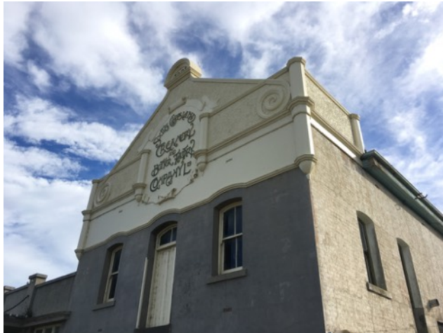
Figure D4. Blue area J. The upper level of the south elevation of the 1908-09 building. Note the skilled craftsmanship of the highly ornamental decorative gable end and parapet which wraps around the corner of the east and west elevations. The original joinery of the doors and windows is intact. The Federation Anglo-Dutch design with Art Nouveau writing is a unique, fine and intact example as there are no other known examples on butter factories in Victoria. The architects designed Art Nouveau writing on plaques on other buildings but these are mainly in the Western District and arguably this is the best example.
