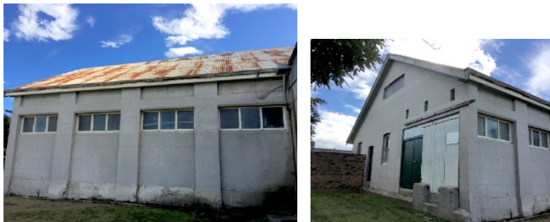
Figure D11. Area G. Left: South elevation of the c1931 factory extension, divided into four bays by pilasters, with highlight windows, and rendered to match the 1931 office building adjacent. Right: The rendered gable end of the single storey extension. The north elevation walls are built of brick with some corrugated iron cladding See Figure D2.
