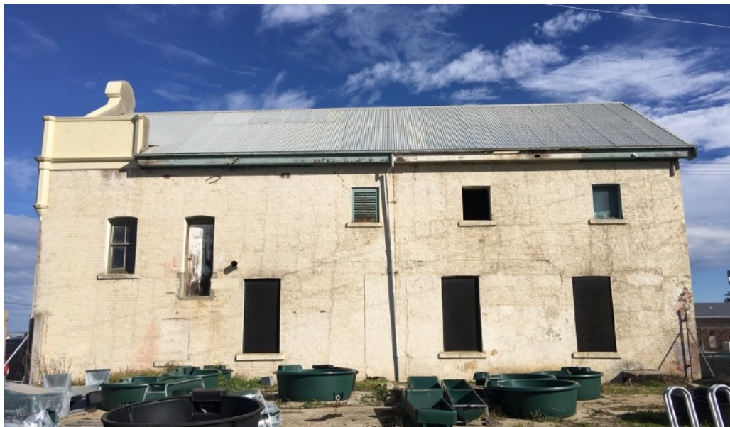
Figure D3. Blue areas A, B, H, I, J. The east elevation has a good degree of integrity. Figure D3 shows the gabled roof clad in galvanized iron and the red brick wall 'bagged'. Segmentally arched openings are located towards the front section. The first floor left hand window is original, the next one has been altered to be a doorway. Two small windows have been bricked up. Towards the northern end of the wall, at first floor level, are three square openings with flat arches, one of which has timber louvres and it is likely that they all had louvres. At ground level are three large flat arched window openings which have been temporarily blocked up on the inside and one that has been infilled. All the openings, except the altered doorway, have projecting sills as seen on the south facade and all of these openings date from 1908-09. The spouting has corroded and is allowing water to soak around the base of the building, most likely contributing to the uneven settling and minor cracking.
