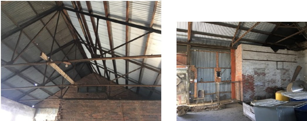
Figure D14. Area G. Left Typical view of the gabled roof of the single storey c1931 factory, with metal roof trusses and galvanized corrugated iron cladding and brown brickwork. Right. View showing red brickwork and corrugated iron walls. The brown brick sections may be earlier remnants of pre 1931 structures.
