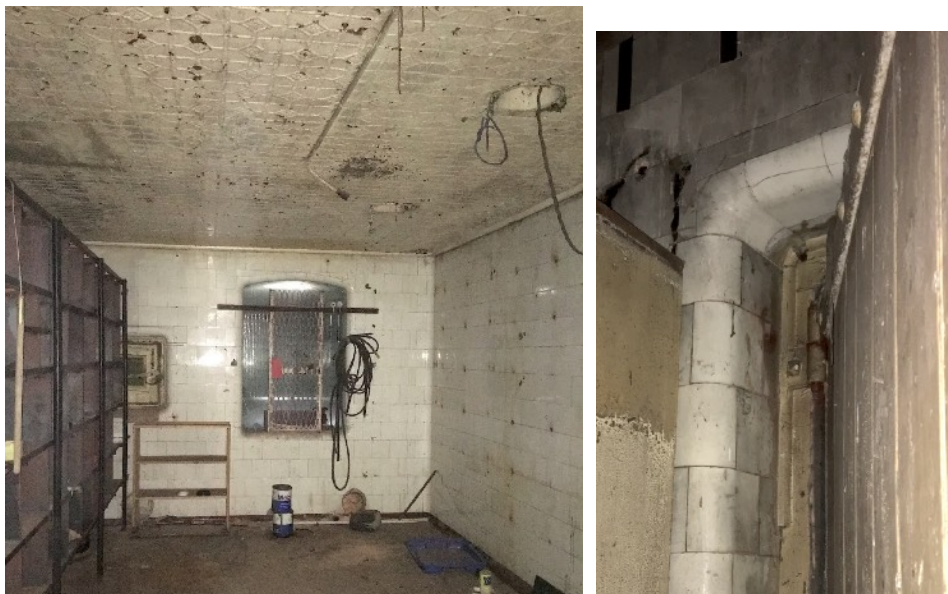
Figure D8. Area C. Looking south to the intact white glazed wall tiles, red-brown hexagon floor tiles, pressed metal ceiling, small hatch, and window and the door opening lined with curved tiles.
