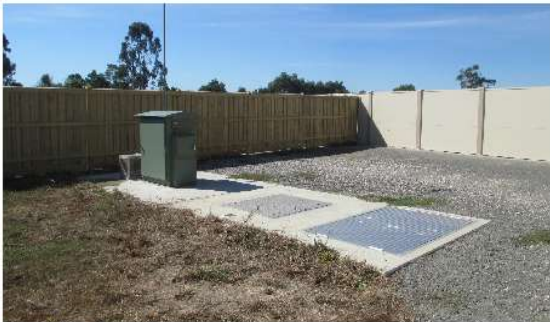
Gaston Trafalgar Pumping Station
