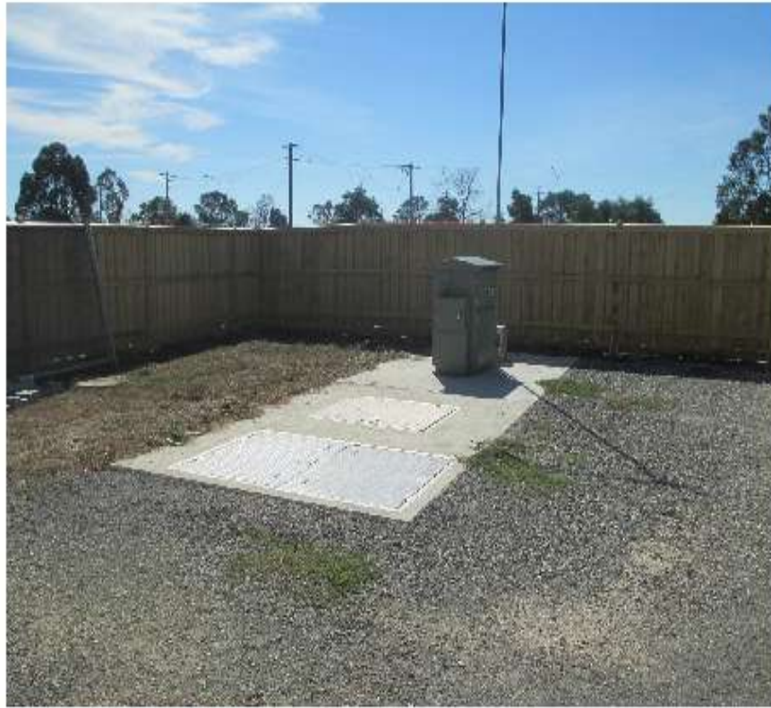
Gaston Trafalgar Pumping Station
