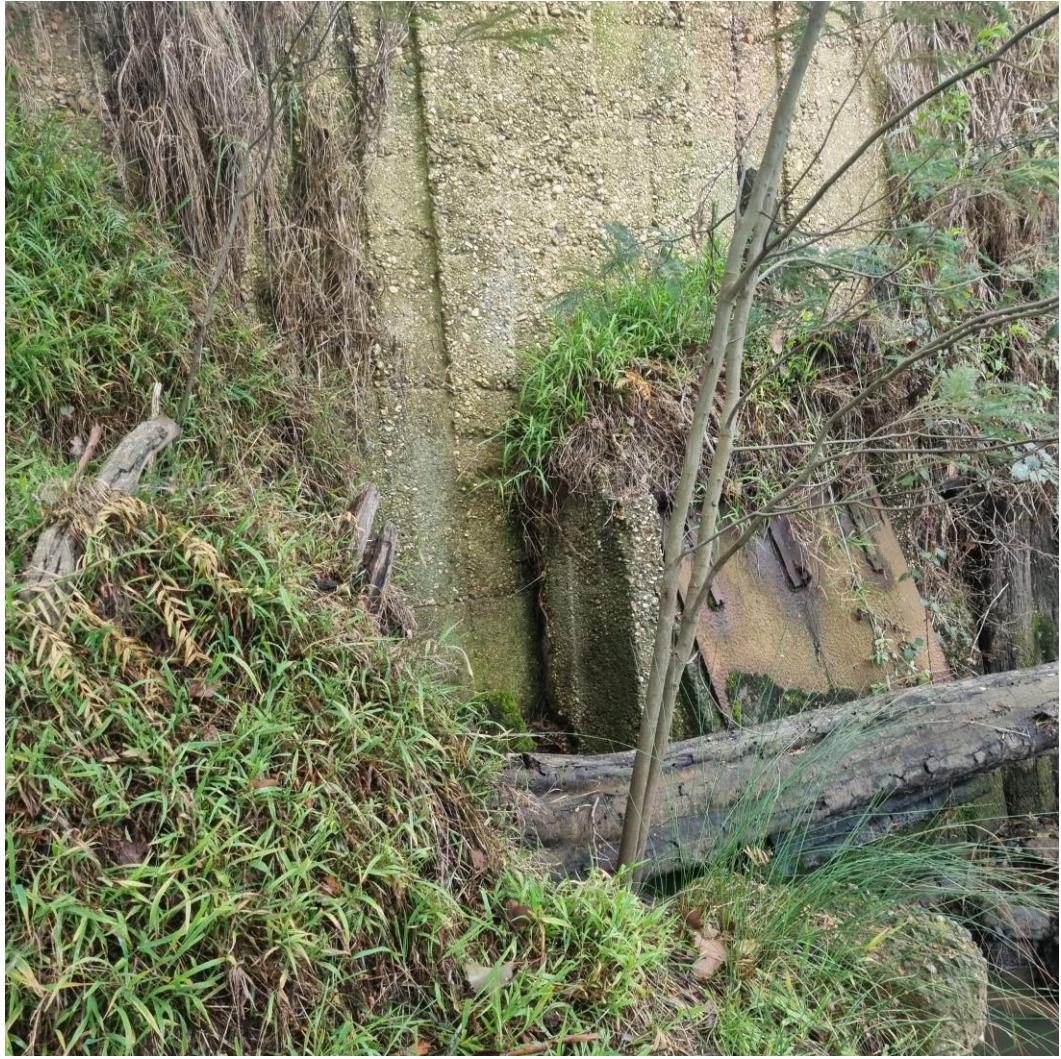
Figure 40. Pipe Connection through high point
